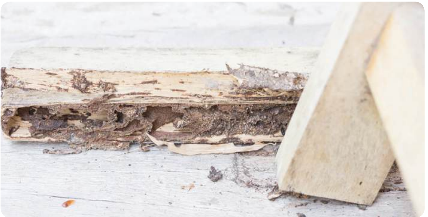
Typical Termite Damage
