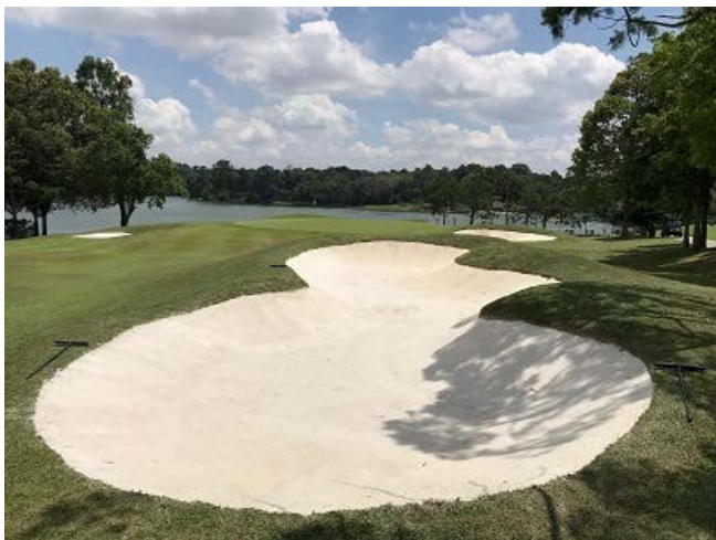
Installation of Capillary Concrete at the greenside bunkers on the sixth hole of the SICC’s Island Course has ‘significantly improved bunker playability, particularly after periods of heavy rainfall’.
