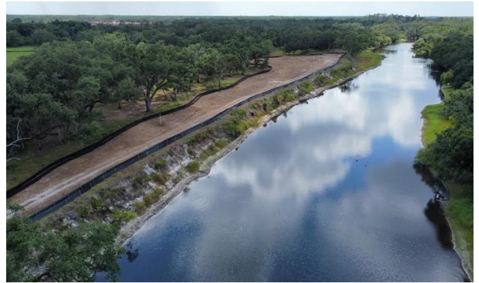
A par 3 under construction at Miakka Golf Club sits along the Myakka River in Florida. (Jason Lusk/Golfweek)
